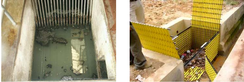
Figure AX2.5: Primary Outlets Clogging
