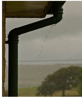
Figure AX2.3: Leaking Downpipe
