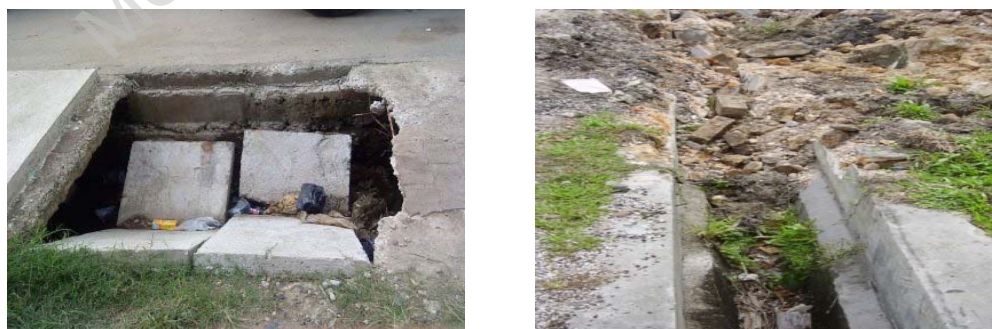
Figure AX2.7: Structure Failure
