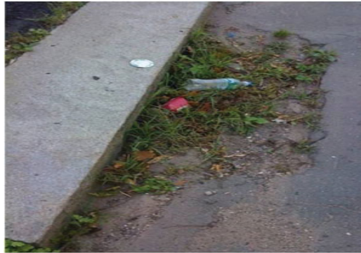
Figure AX2.9: Clogging Inlet
