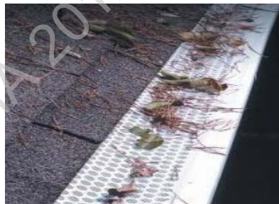
Figure AX2.2: Partially Clogged Gutter Screen
